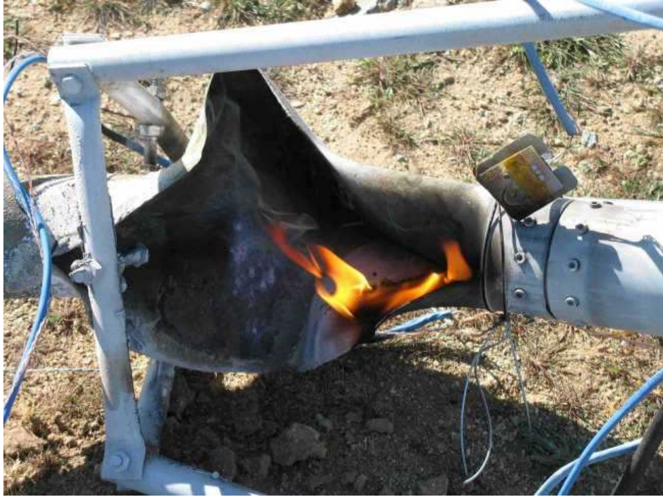
Photo 6 – Ruptured 1 st phase casing aft of mid-bulkhead
